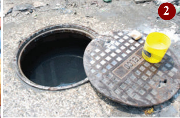
Manhole kept open on a road
