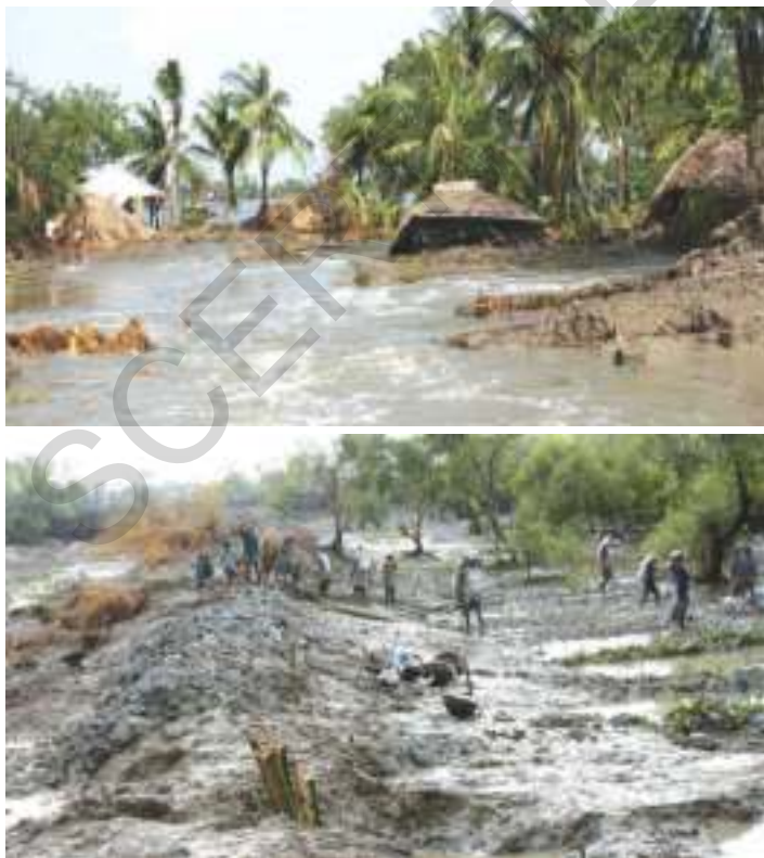
Fig 4.4 : Impact of Aila : (Top) broken embankment, (Bottom) repairing embankment
